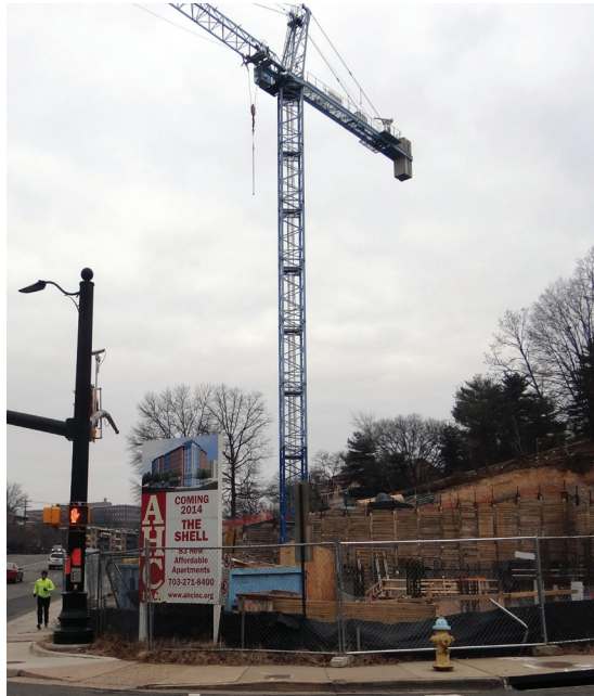
The Shell, AHC, Inc.'s new construction along Columbia Pike, takes advantage of “contingent land” belonging to AHC’s Harvey Hall to increase density, permitting 83 committed-affordable units to be built.
